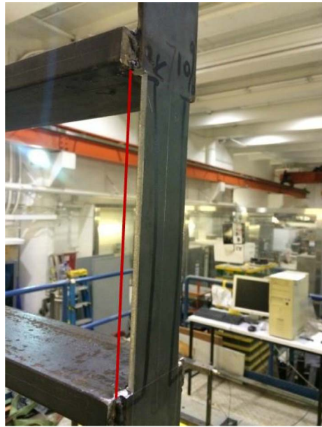
(b) Introduced damage at the 7th floor (20% reduction of cross section area of one column)
