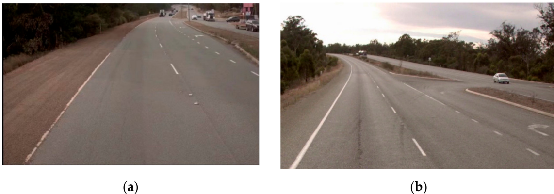
Figure 1. Examples of pavement markings in poor condition. (a) Edge line (left side) is worn down and even missing; (b) turning arrows and continuity line (right side) are blurred.
