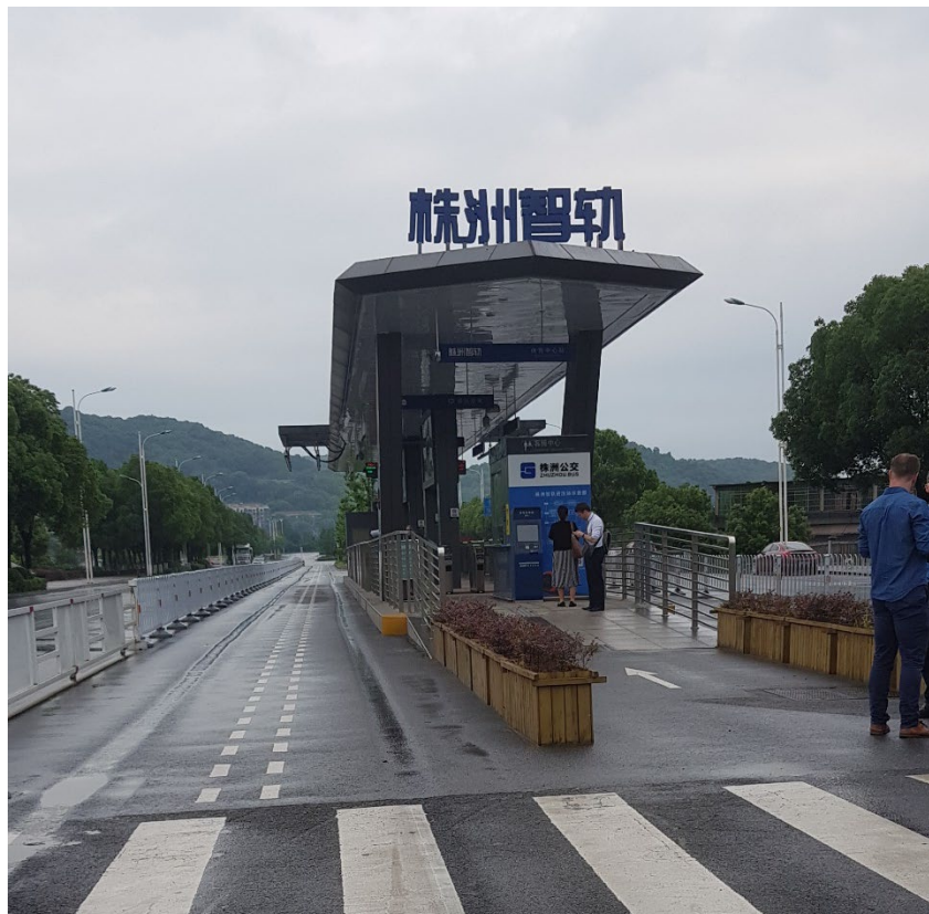
Zhuzhou pavement deformation at ART station
