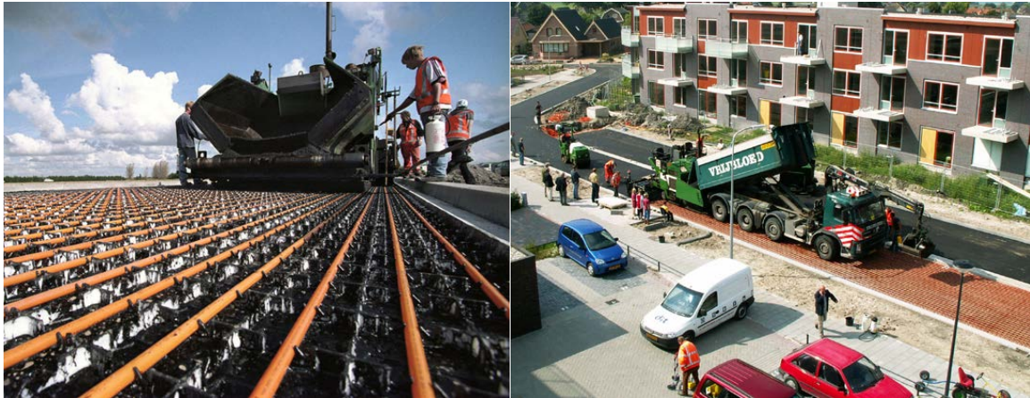
Figure 3: The use of pipework to extract heat from road surfaces in the Netherlands.
