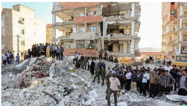
Figure 1: An example of construction waste accumulation after an earthquake in Azgaleh, Kermanshah, Iran 2017.
