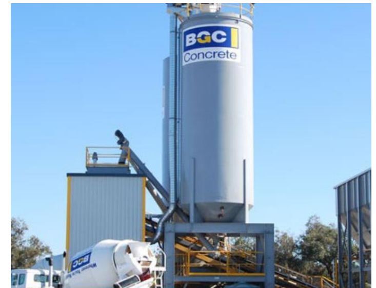
Dedicated silos with granulated blast-furnace slag
