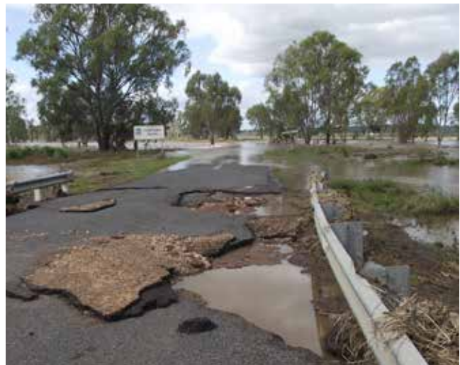
The damage to roads caused by storms. Image: Queensland Department of Transport and Main Roads, 2012.
