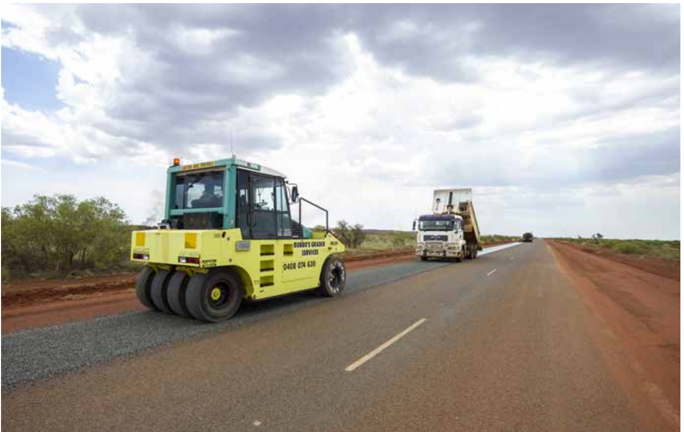
Road maintenance being carried out in a rural area. Image: Main Roads Western Australia, 2012.
